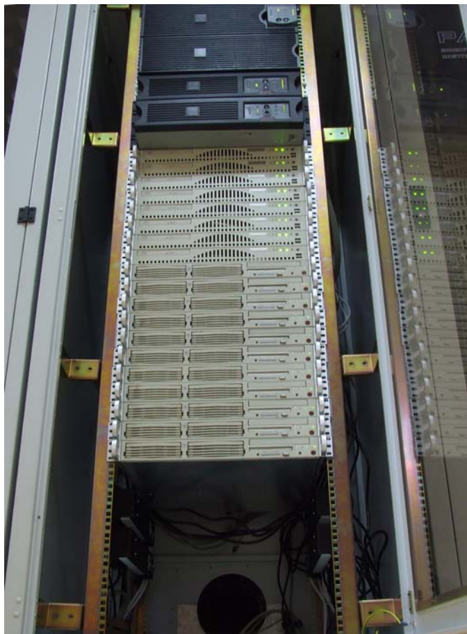
Figure 2 – No. 3 Rack with Worker nodes
